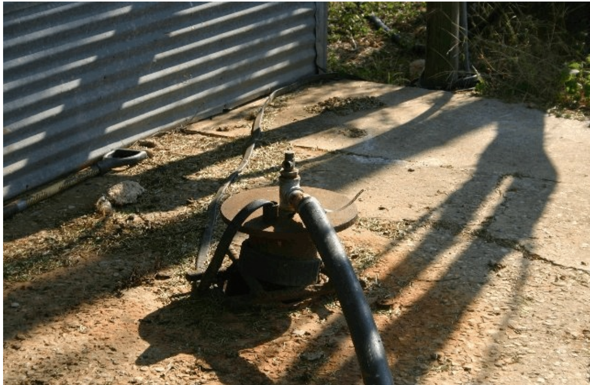
VIEW OF WATER WELL
